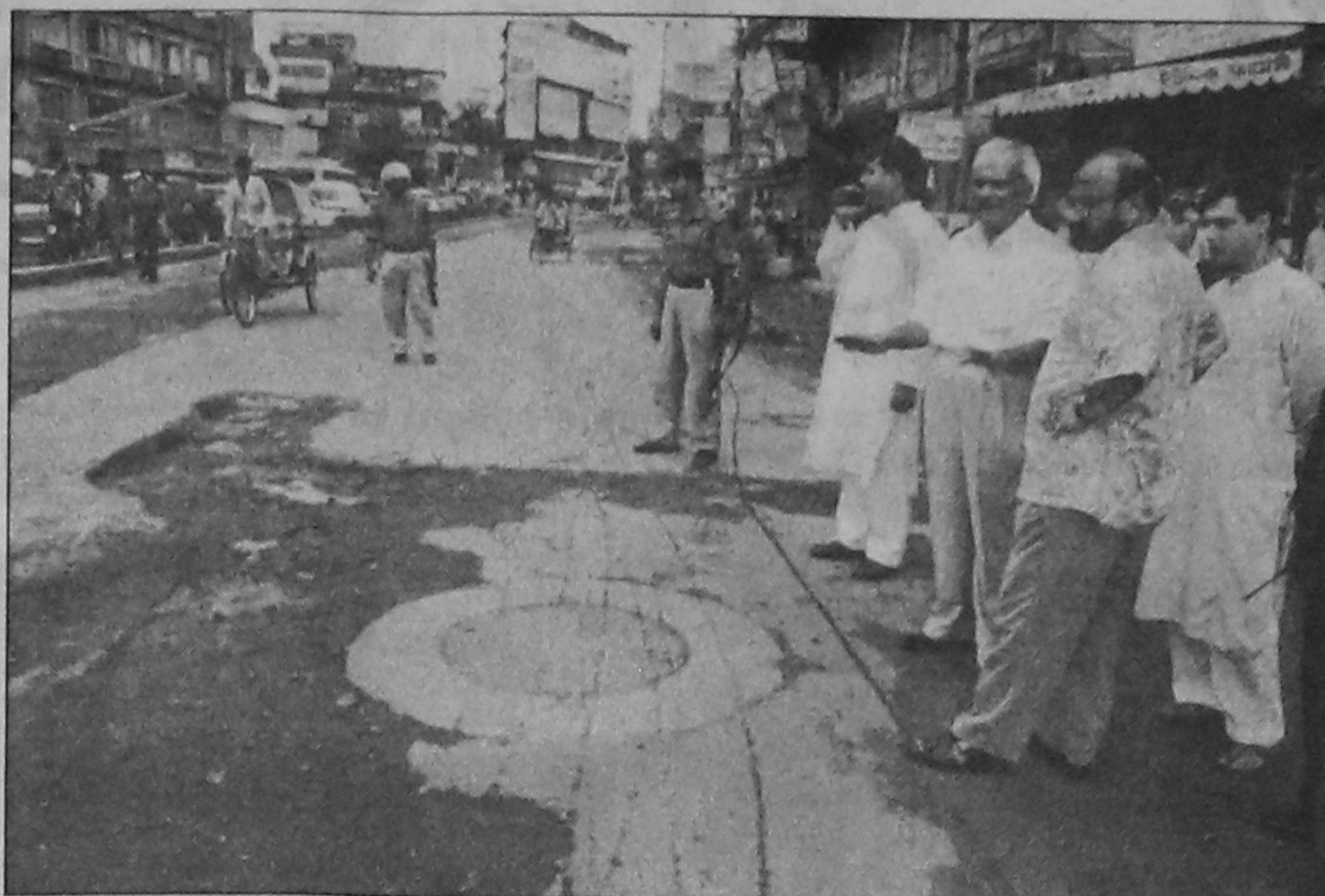
DCC Mayor Sadeque Hossain Khoka visited different areas of the city yesterday to see the condition of the roads.
