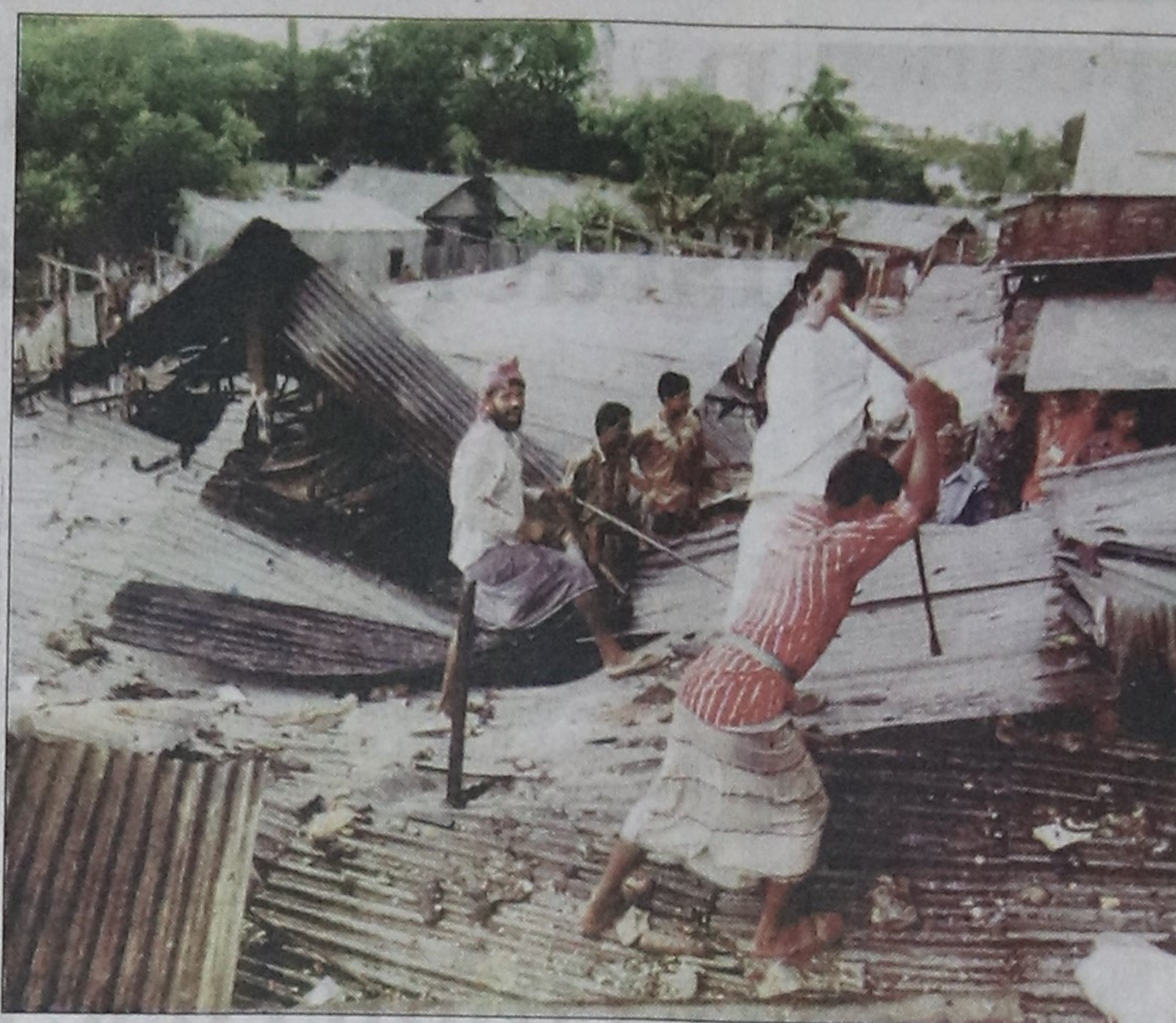
Workers dismantle shanties erected on the land of T & T Board in Malibagh area of the city yesterday as part of the eviction drive against the illegal occupiers.
