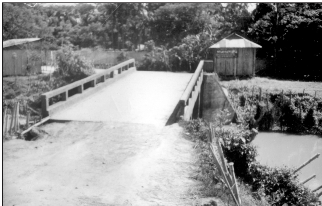
A portion of a pucca bridge on Nabiganj-Innatganj Road has been collapsed due to poor quality of work and bad condition of the approach.
