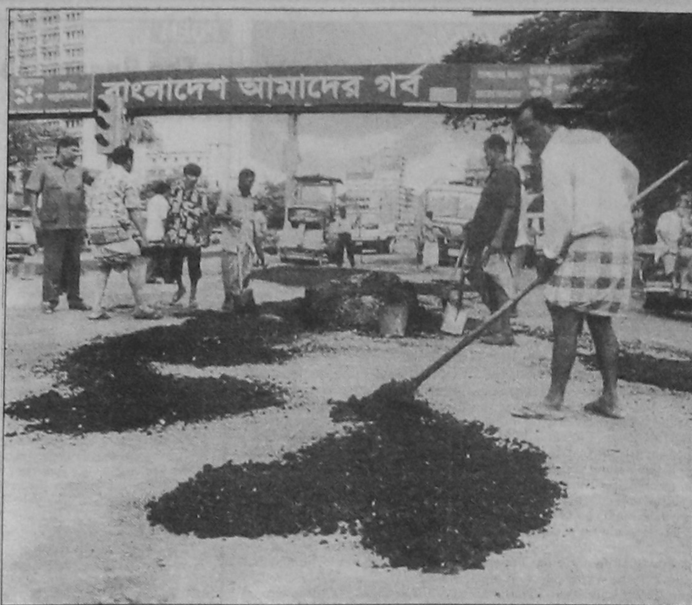
Workers repairing a road near Muktangan in the city yesterday (left) whereas other pothole-strewn roads, such as this road (on the right) near Dhaka Zila Parishad office, which need immediate repair, have been left as they are for long.
