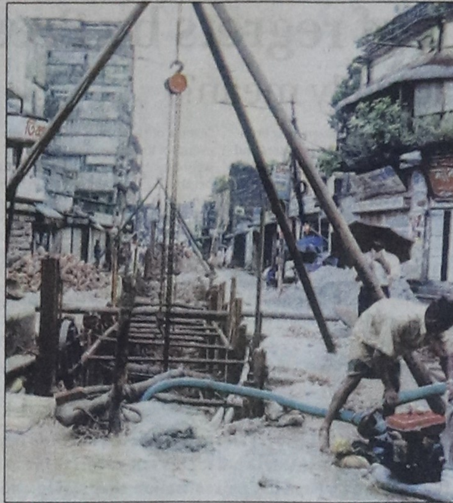
PHOTO STAR Road digging continues in Nawabpur area in the city despite a DCC ban on it during the monsoon. As a result, the road users suffering a lot but the authorities remain indifferent.
