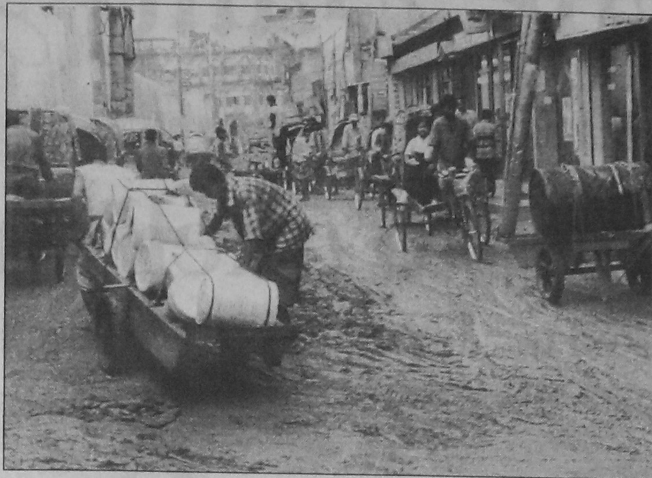
Pothole-strewn Nazimuddin Road poses a road hazard to the pedestrians and the passengers as well. This road has been in very bad shape for long but the authorities remain indifferent to the woes of the road users.
