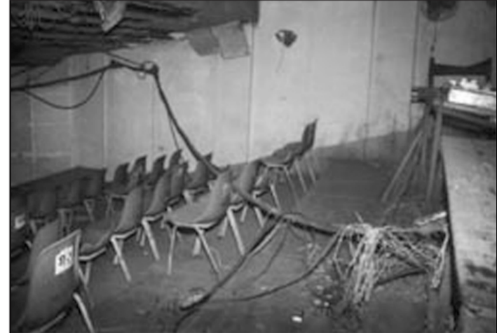
Bare electrical wiring behind viewers at balcony of Guide House
