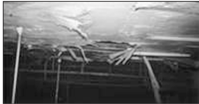
Guide House auditorium ceiling in alarming condition
