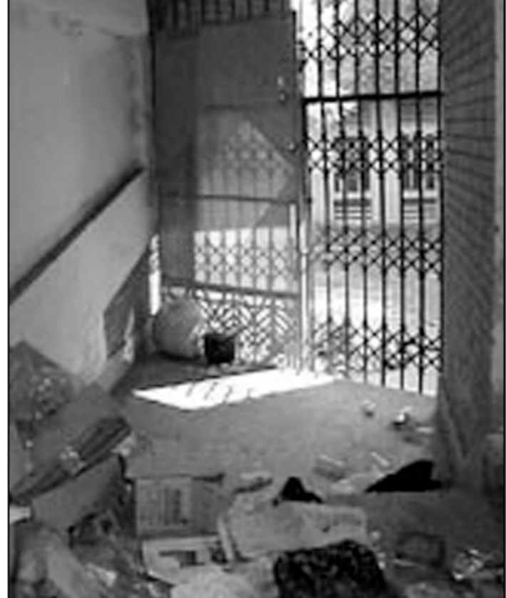
Public Library secondary exit has become a waste dump and remains closed during show time.
