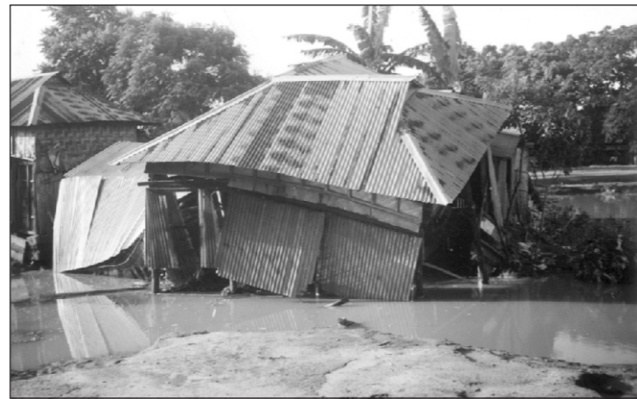
(Left) A flood damaged house at Goshgoan bazaar of Dhubaura upazila in Mymensingh, (middle) another flood affected kutcha house at village Pancha Nandapur in Mymensingh and (right) erosion affected Kamarjani area in Gaibandha due to flash flood.
