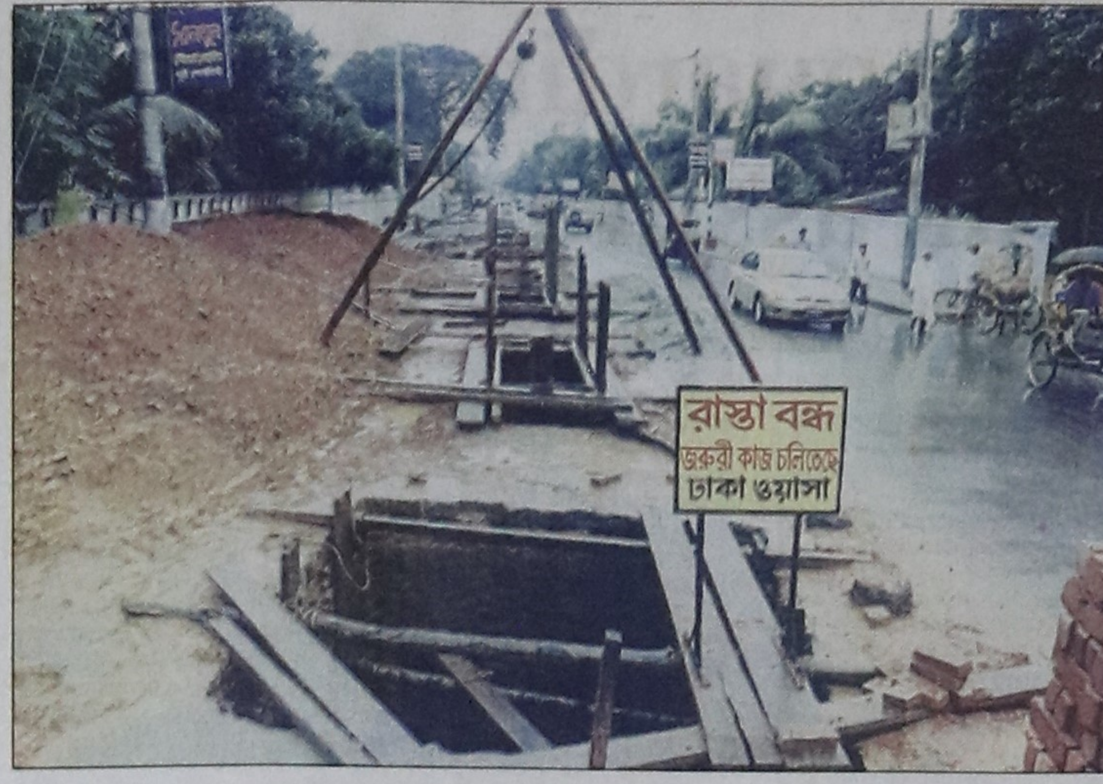
The Dhaka WASA runs its installation work on the Holy Family Red Crescent Hospital Road despite the DCC's ban on road-digging in monsoon.
