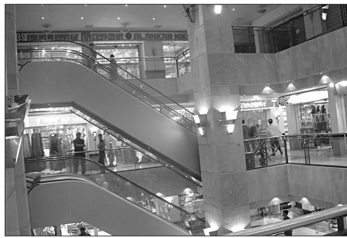
No provision to enclose the escalator to restrict the spread of fire.
