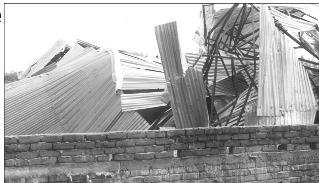
A cyclonic storm damaged tin-shed house of Amodpur College in Pirganj upazila in Rangpur. Total loss of the college caused by the natural calamity has been estimated to be Tk four lakh. Furniture and other valuables of the institute have been completely damaged due to the storm which lashed recently over the entire Rangpur district.
