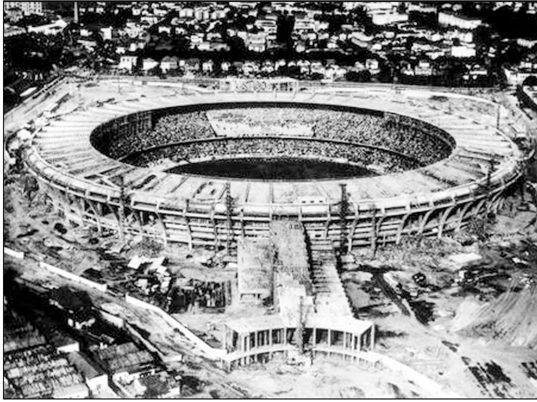
Aerial view of the Maracana Stadium, still under construction at the time of the kick-off of the 1950 FIFA World Cup Brazil. The Brazilian authorities had decided to build the biggest stadium in the world with a capacity of 220,000, but the work schedule, begun in 1948, proved unrealistic, so the competition got underway in an unfinished stadium.
