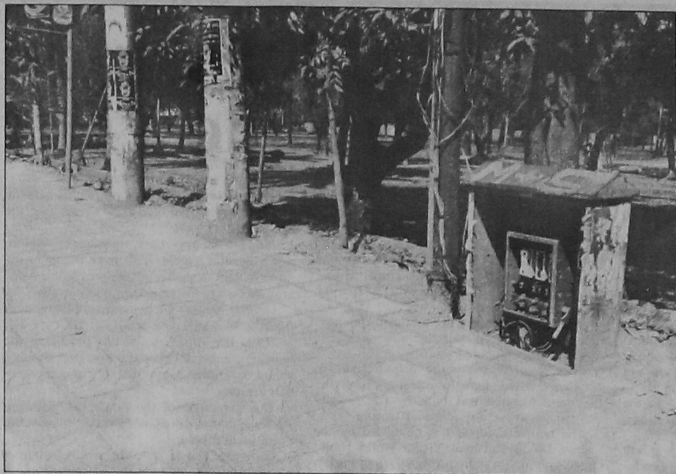
An open electric switch box poses potential risk for the passers-by as it is located just on the edge of a footpath opposite to the central library of Dhaka University.
