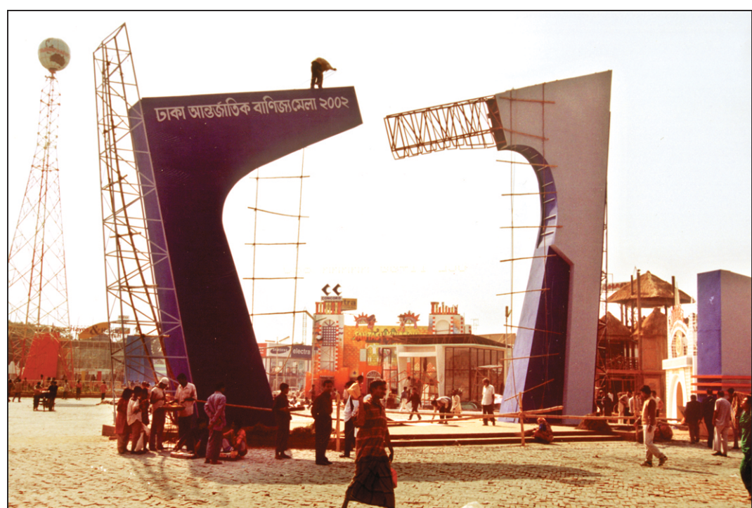
Although the DITF opens today, a lot of work inside the fair ground and construction of the entrance gate remained unfinished yesterday.
