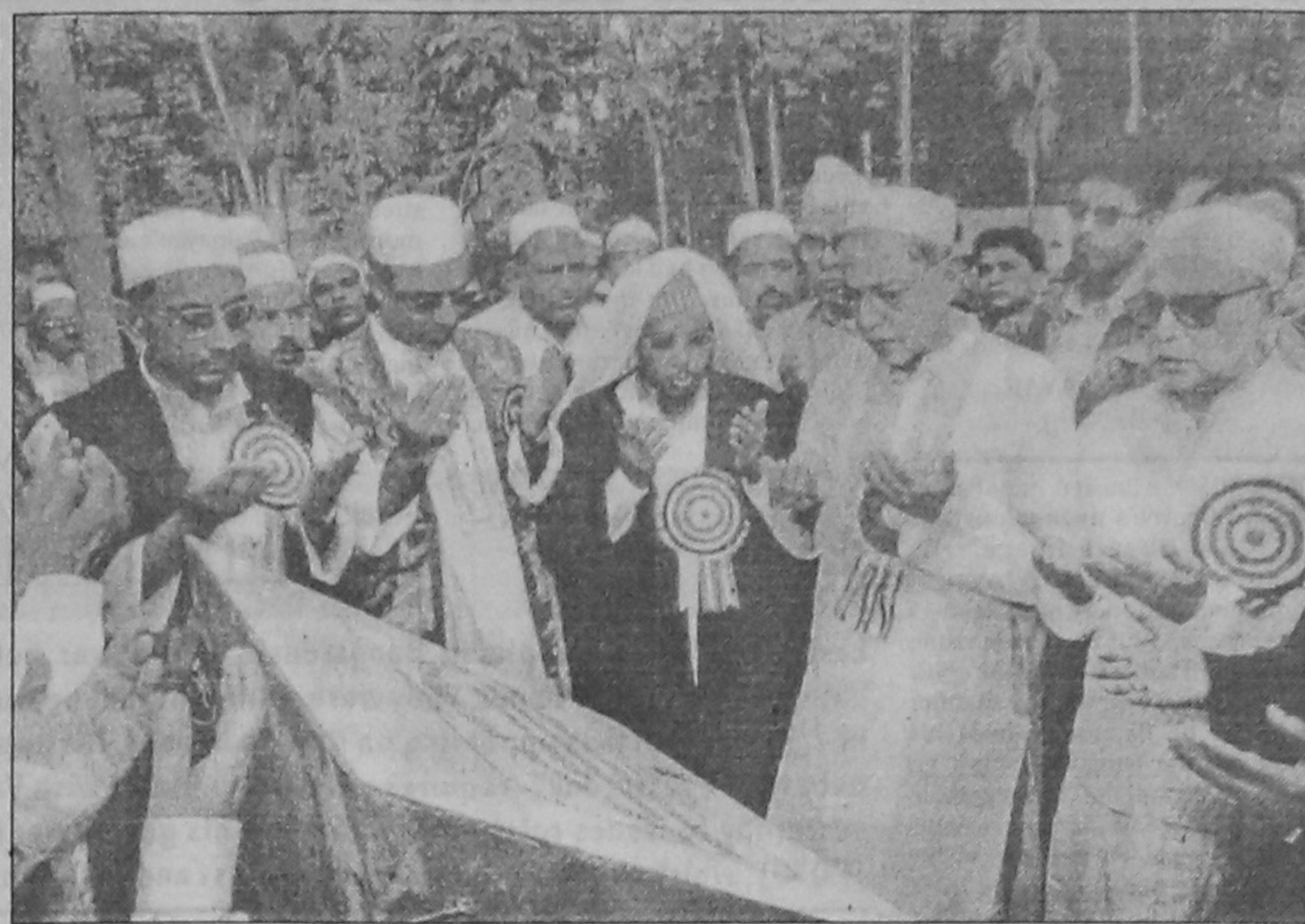
President A.Q.M. Badruddoza Chowdhury offering munajat after laying the foundation for reconstruction of Dhanmondi Eidgah Jame Mosque in the city yesterday.
