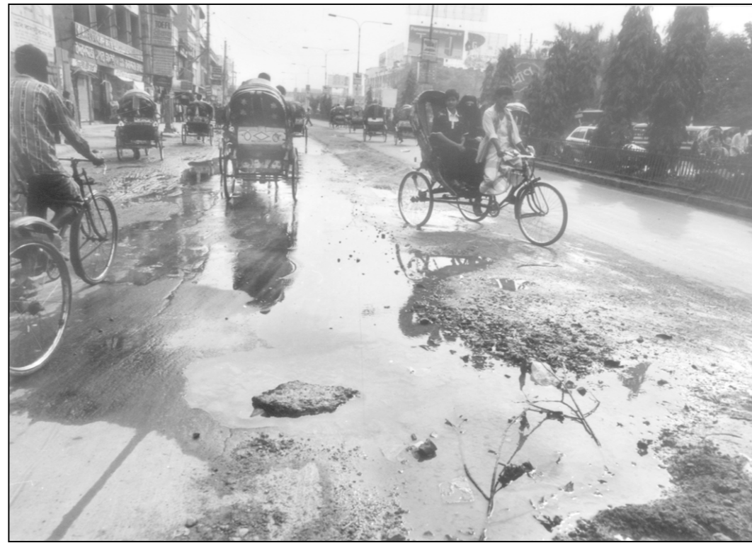
Water overflowing city roads, Mirpur Road in front of Dhaka College, a case in point, because of leakage from WASA pipes is an all too familiar sight.
