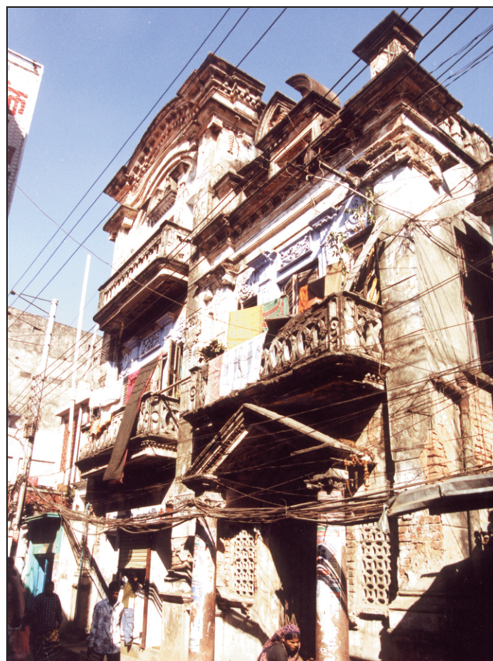
Seismic shock...any earthquake with high magnitude may knock down many old rundown buildings like this (in the picture), which dot the cityscape of Old Dhaka.
