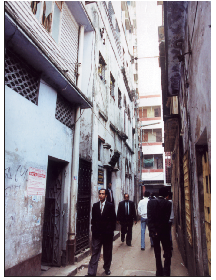
This house (right) at 31 Court Street in Kotwali in the city slightly tilted during the mild tremor in the country on Wednesday.
