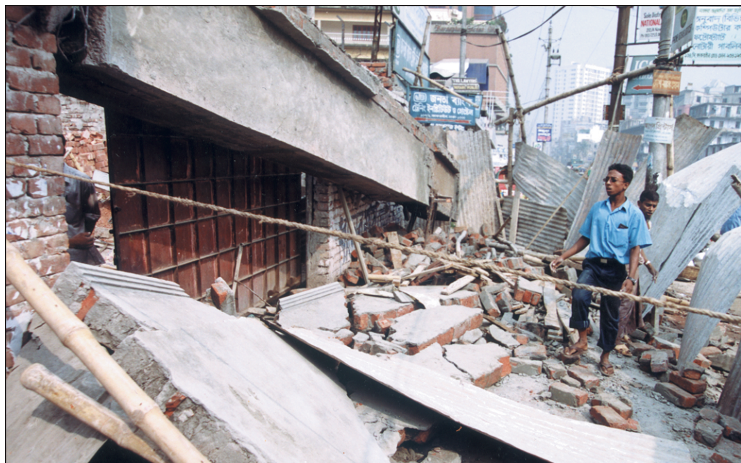
A beam of the first floor of an under-construction building collapsed in the city's Kakrail area yesterday, killing a mason and injuring a helper on the spot.
