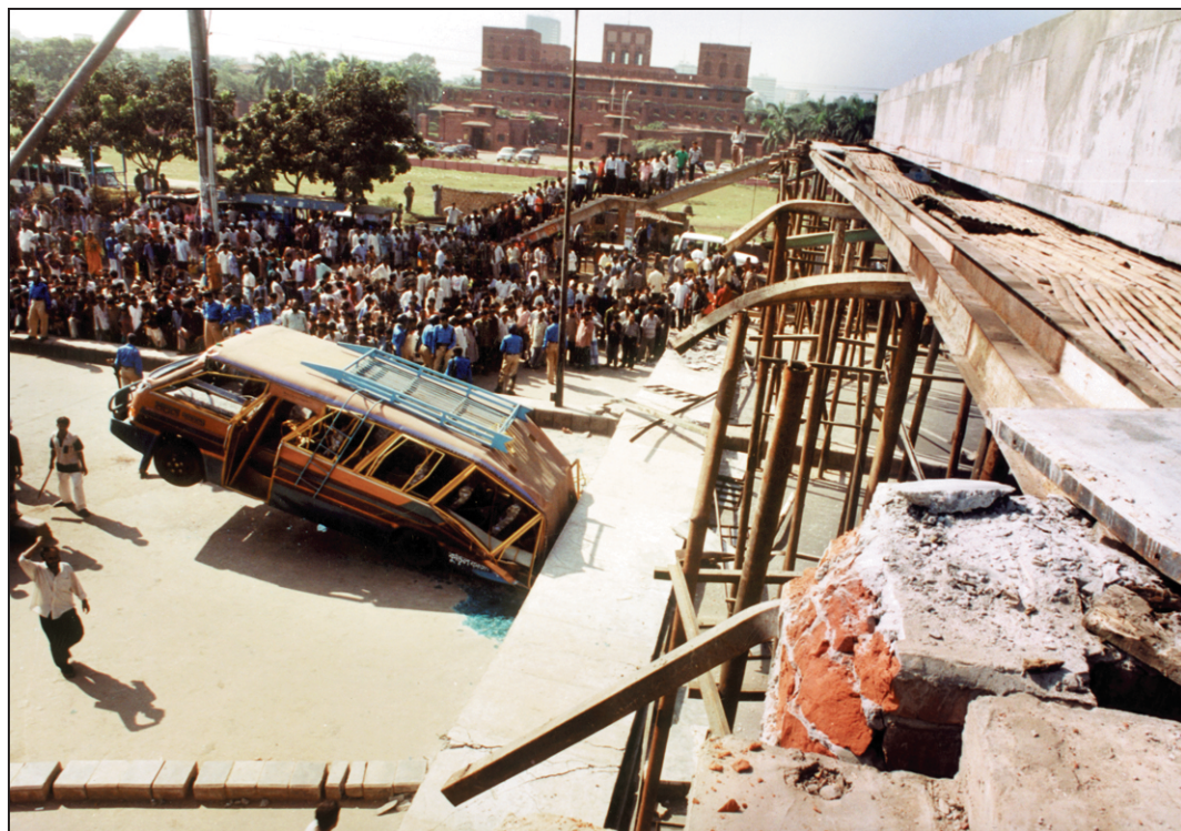
Police are on guard against curious onlookers on the scene where an under-construction footbridge crumbled on a passenger bus near the US Embassy at Baridhara yesterday.
