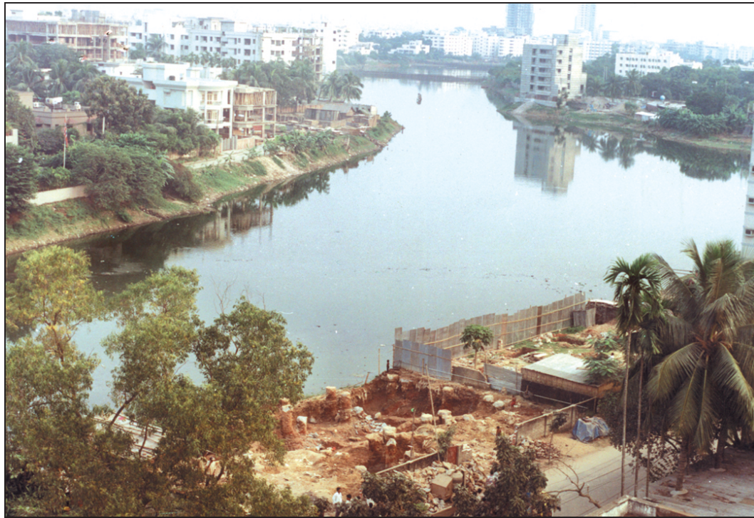
Unplanned urbanisation... construction work for two bridges over the Gulshan-Banani-Baridhara Lake in the city, endangering the water body further.
