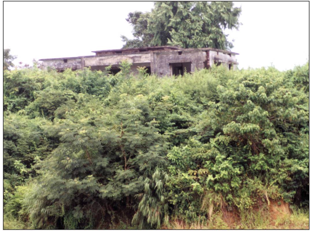
PHOTO: A K M MOHSIN Abandoned Balukhali Union Parishad Bhaban in Sadar thana of Rangamati hill district. Members of former Shanti Bahini blasted bombs and damaged this building situated on a hillock in 1984. After three years of signing of Chittagong Hill Tracts (CHT) Peace Accord this union parishad building under local government still remains the same.
