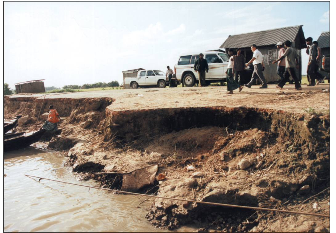
Unabated river erosion at Arial Khan ferry ghat (terminal) in Madaripur. Immediate measures should be taken to check the perennial problem.
