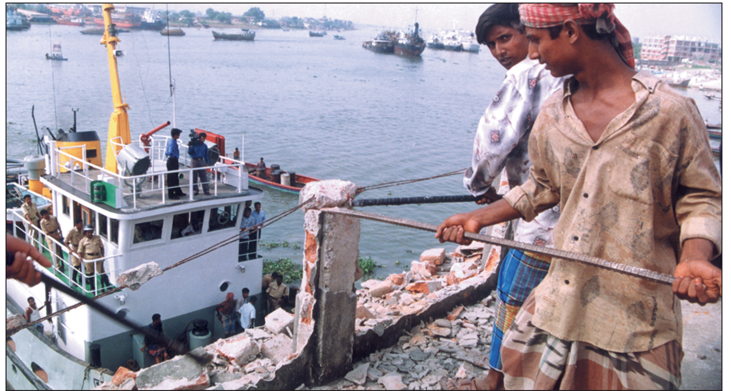
BIWTA yesterday demolished 23 illegal structures along the river Buriganga at Fatullah in Narayanganj. It could not demolish eight such structures due to court order to maintain status quo during the drive to recover foreshore of the river.
