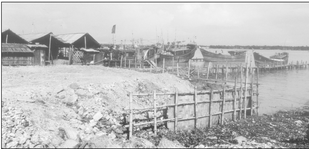
A vicious assault on the river Karnaphuli in Chittagong. A vested group filled up a part of the river at Firingi Bazaar, Yakubnagar Loita Ghat. While the earthfilling continued openly, local administration remained totally oblivious to it. The Karnaphuli has long been subjected to illegal occupation and encroachment, dangerously threatening the ecology of the area.
