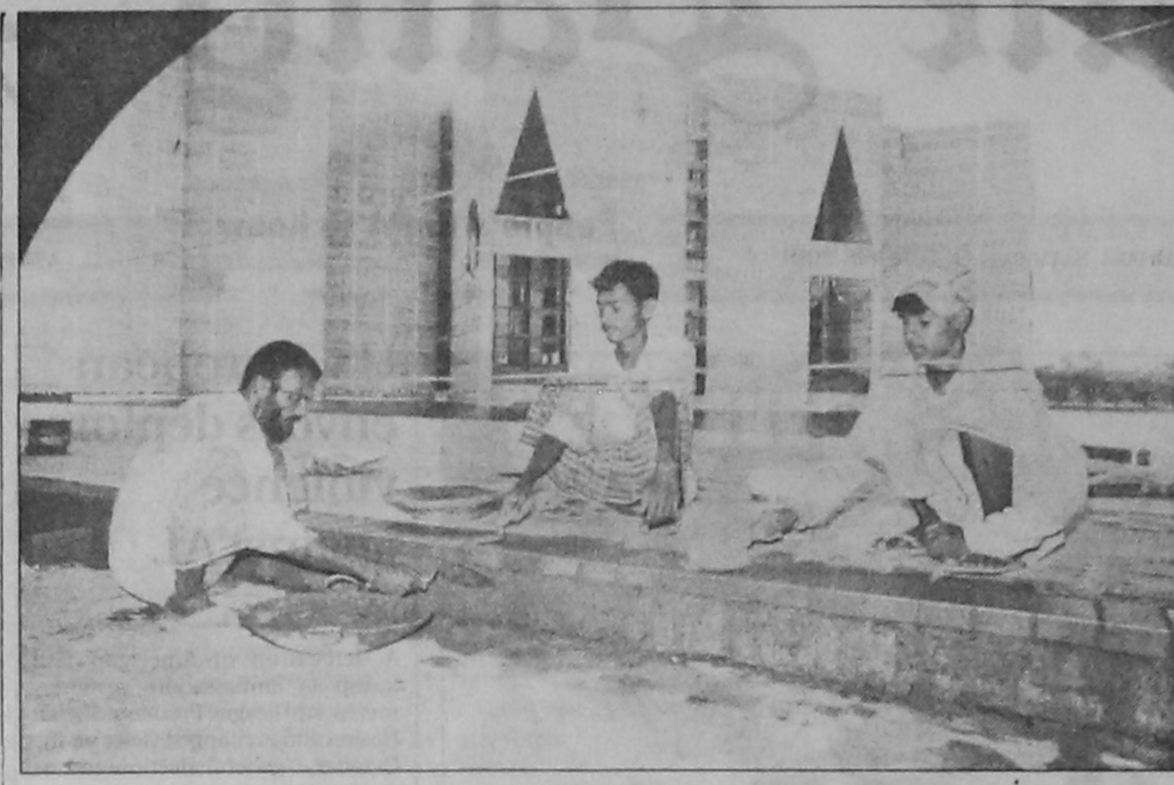
Workers mending the pavement leading to the Jatiya Sangsad yesterday ahead of the oath-taking ceremony of the newly elected parliamentarians tomorrow.
