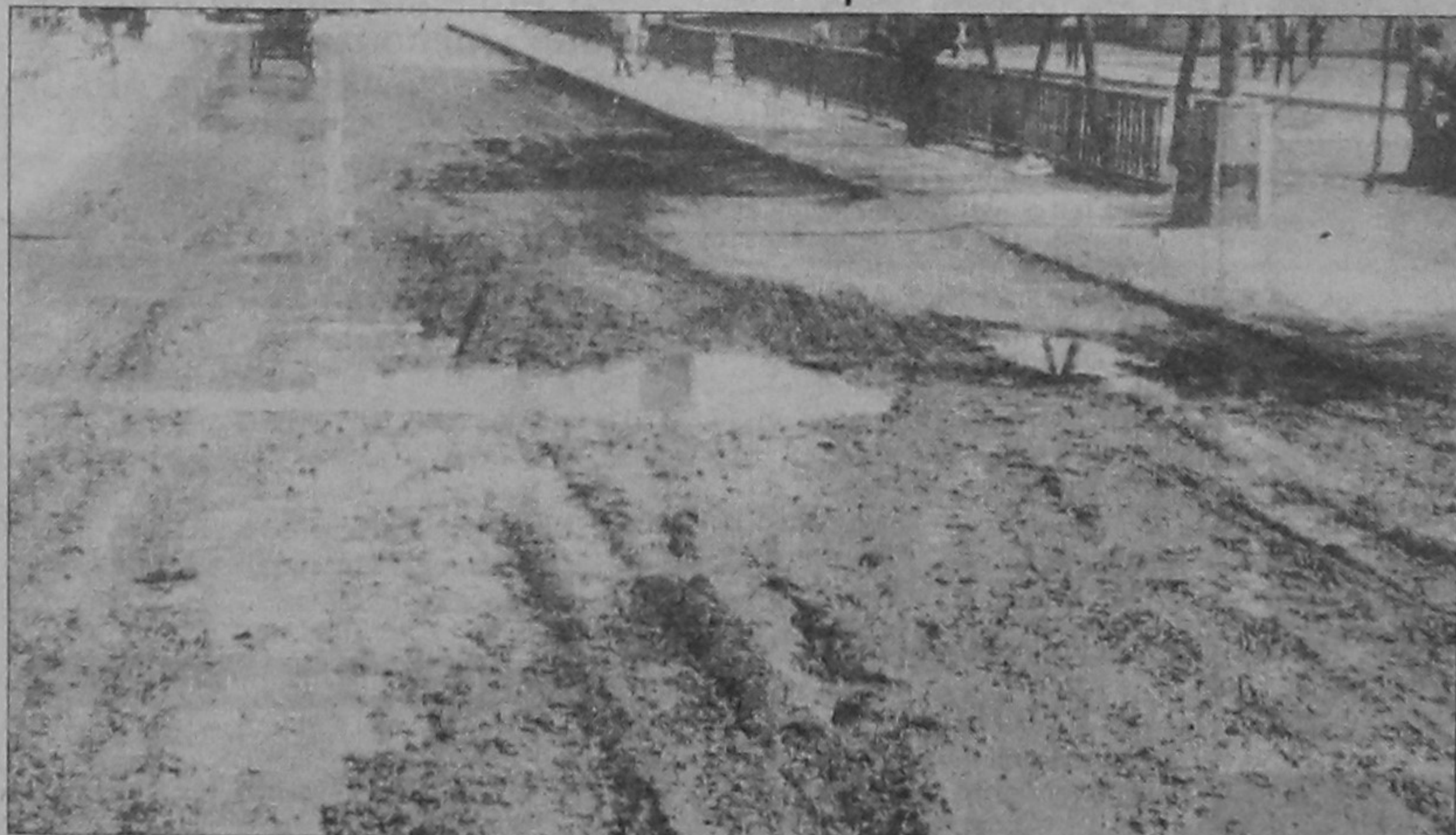
The adjacent road to the second Buriganga bridge is in a deplorable state for quite some time. Due to lack of maintenance and renovation, the road has become unsuitable for smooth traffic and this may lead to serious accidents. For how long people will have to put up with this nuisance?
