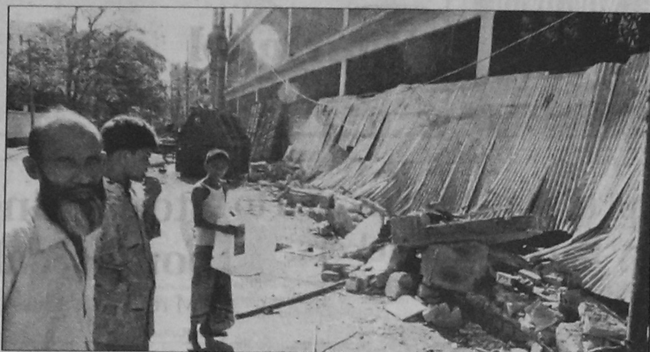
DCC demolished some illegal structures adjacent to the Gulshan No-1 market yesterday.
