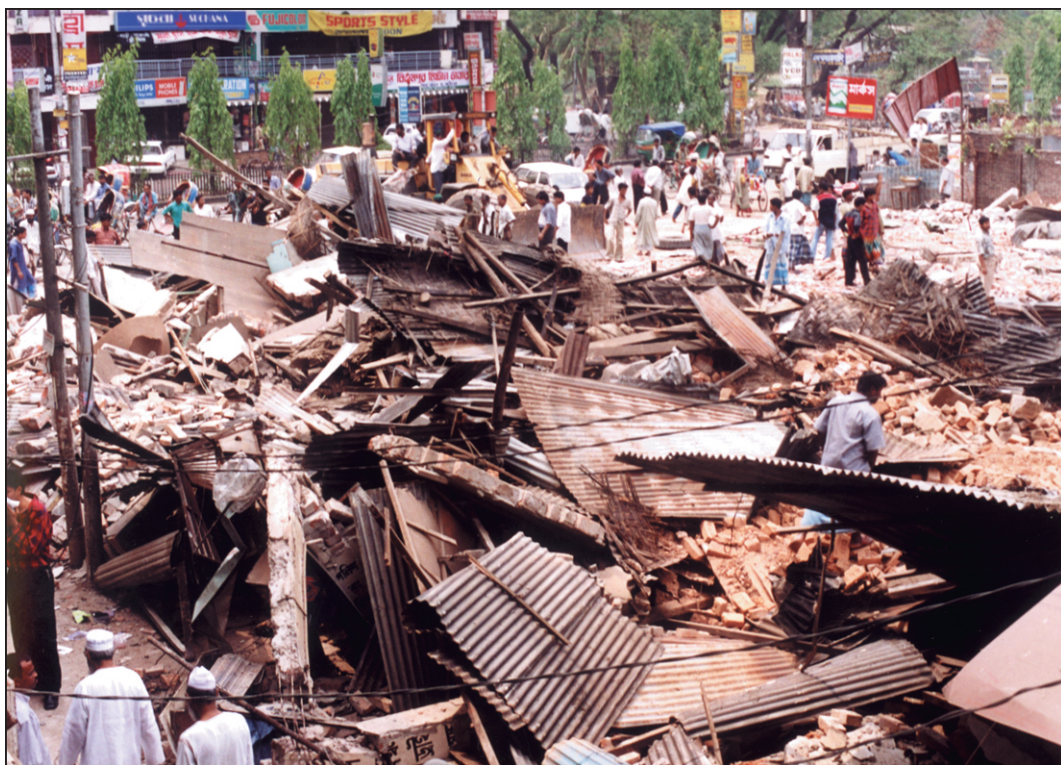
Rajuk demolished two illegal structures erected on a land at Kalabagan in the city yesterday.
