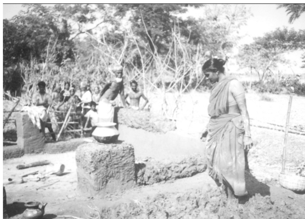
A flood affected woman of Khanpur in Sadar upazila of Satkhira district rebuilding a kitchen which was collapsed along with her dwelling house during last year's devastating flood.
