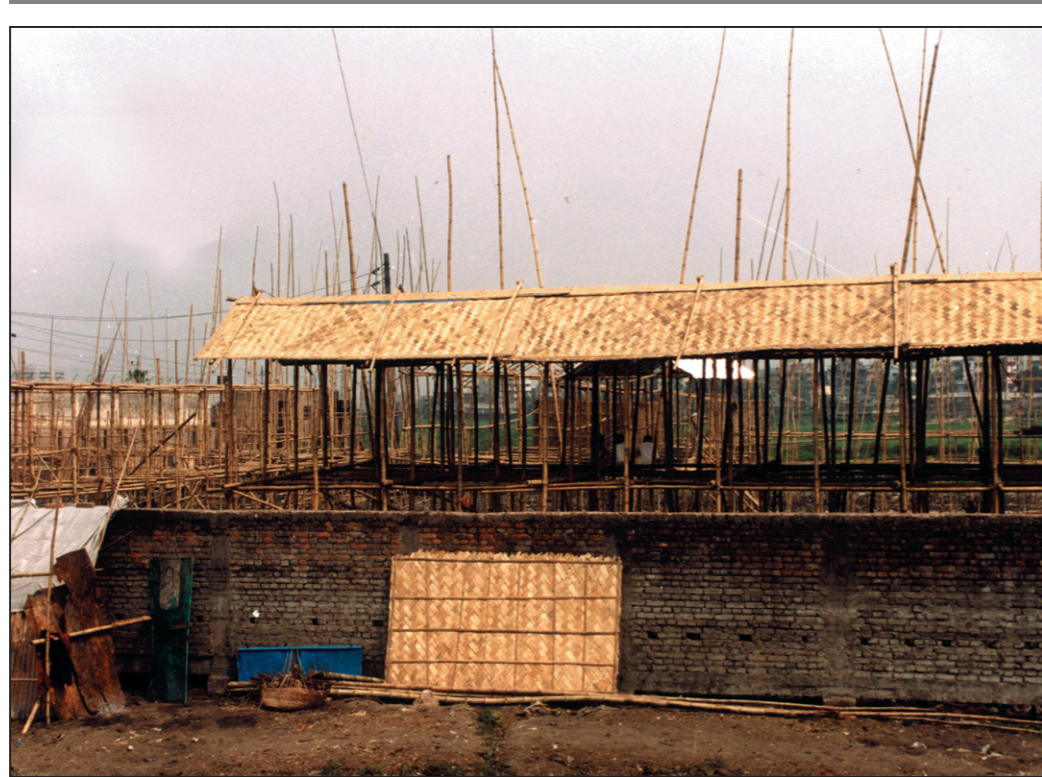
Thatched houses being built less than two months after a devastating fire gutted Bashpatti slum near Moghbazar rail crossing in the city. As the slum regenerates, fresh fears sprout over yet another round of clash over its control that resulted in the fire killing a woman.
