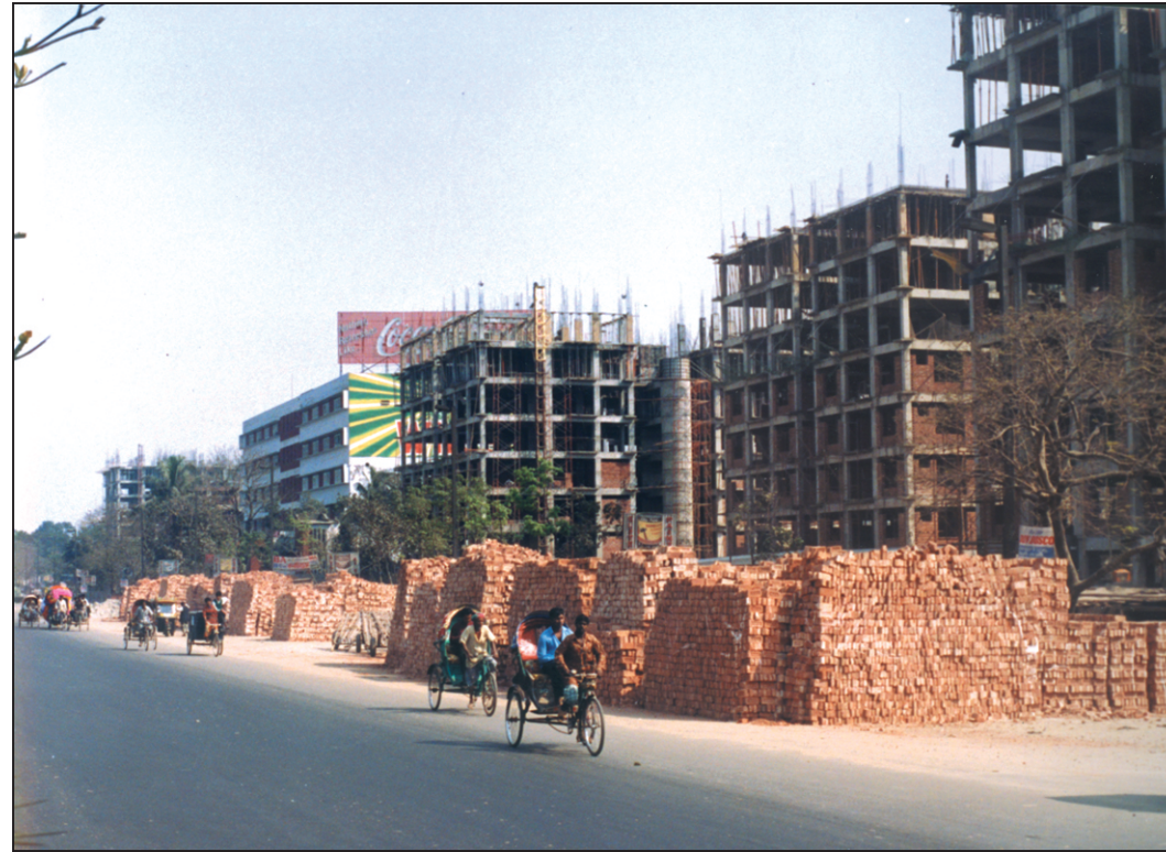
Construction materials occupy a significant portion of the city's Manik Mia Avenue, as work goes in full swing to build apartments for NAM Summit delegates. The buildings are constructed without clearance from the Department of Environment.
