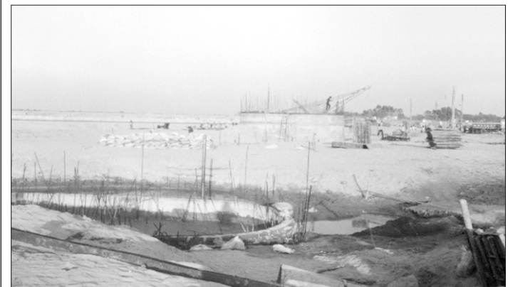
The construction work of Dharla Bridge near Kurigram town is going on in full swing. ---Star photo
