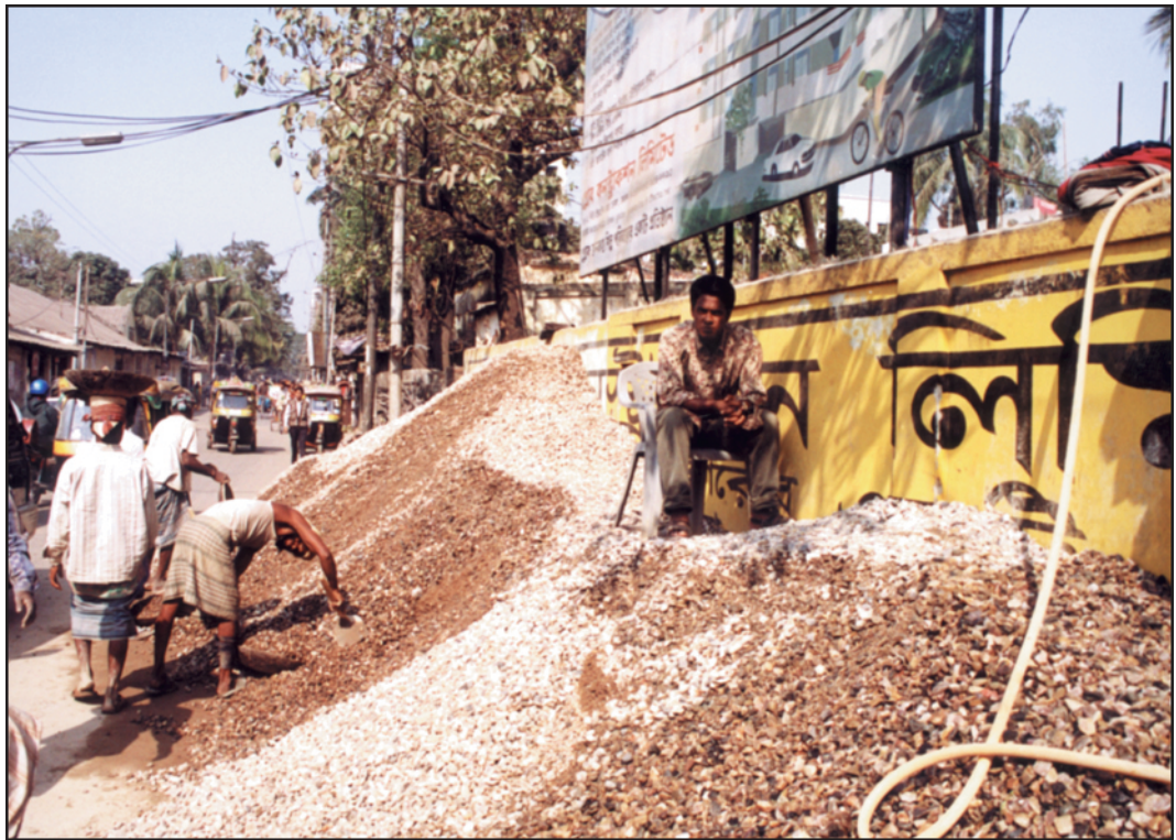
Pedestrians' plight Construction materials piled up on a Segun Bagicha road in the city pose immense inconvenience for pedestrians. The law forbids it, but lack of enforcement lets the offenders get away. -- Star photo
