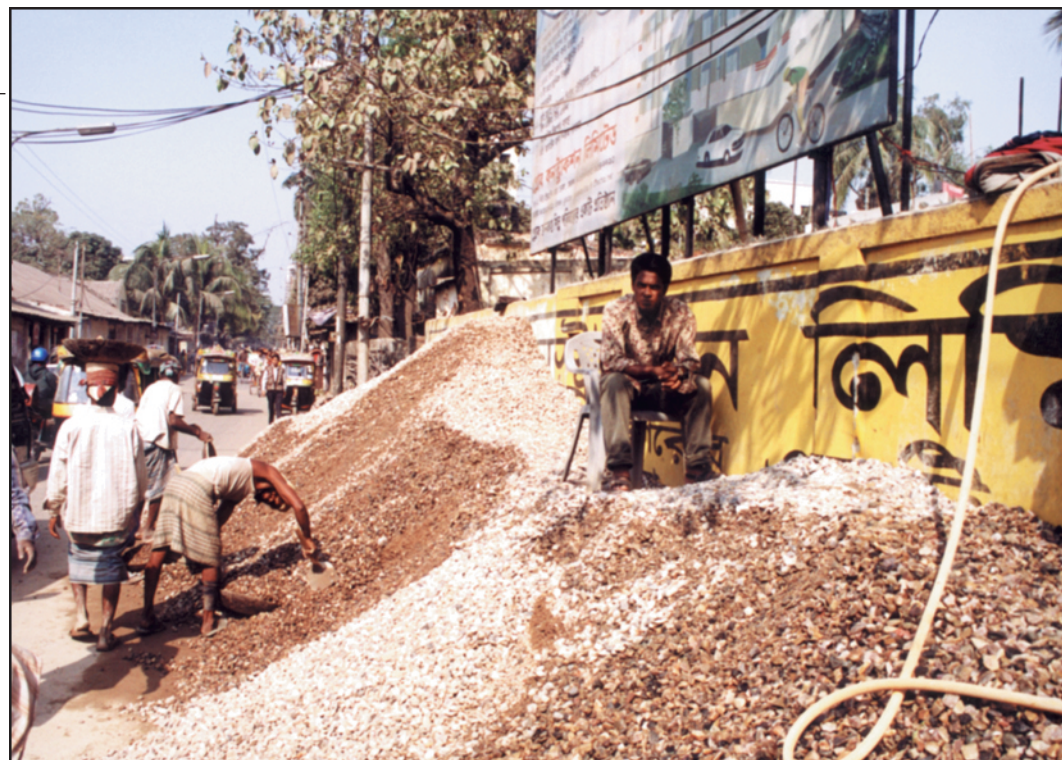
Pedestrians' plight Construction materials piled up on a Segun Bagicha road in the city pose immense inconvenience for pedestrians. The law forbids it, but lack of enforcement lets the offenders get away. --Star photo
