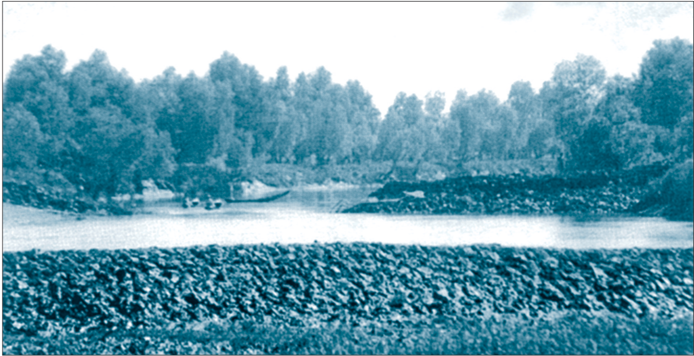
A partial view of an embankment being built by Nasaka, Myanmar's border forces, on the river Naf. BDR and Nasaka traded fire for several hours over construction of the embankment on January 8. -- Star photo by Monayem Khan
