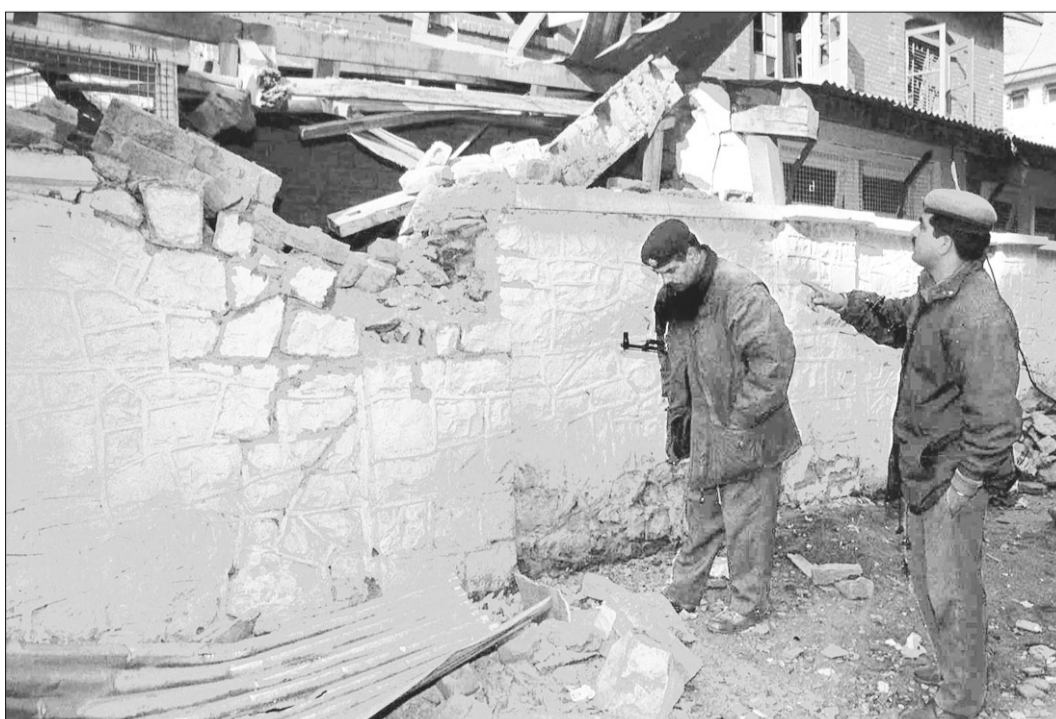
Indian paramilitary personnel inspect a portion of the main telephone exchange in Srinagar that was damaged in a massive explosion yesterday. At least 28 people, including two paramilitary policemen, were injured in a massive explosion, suspected to be the handiwork of Muslim militants. --AFP photo
