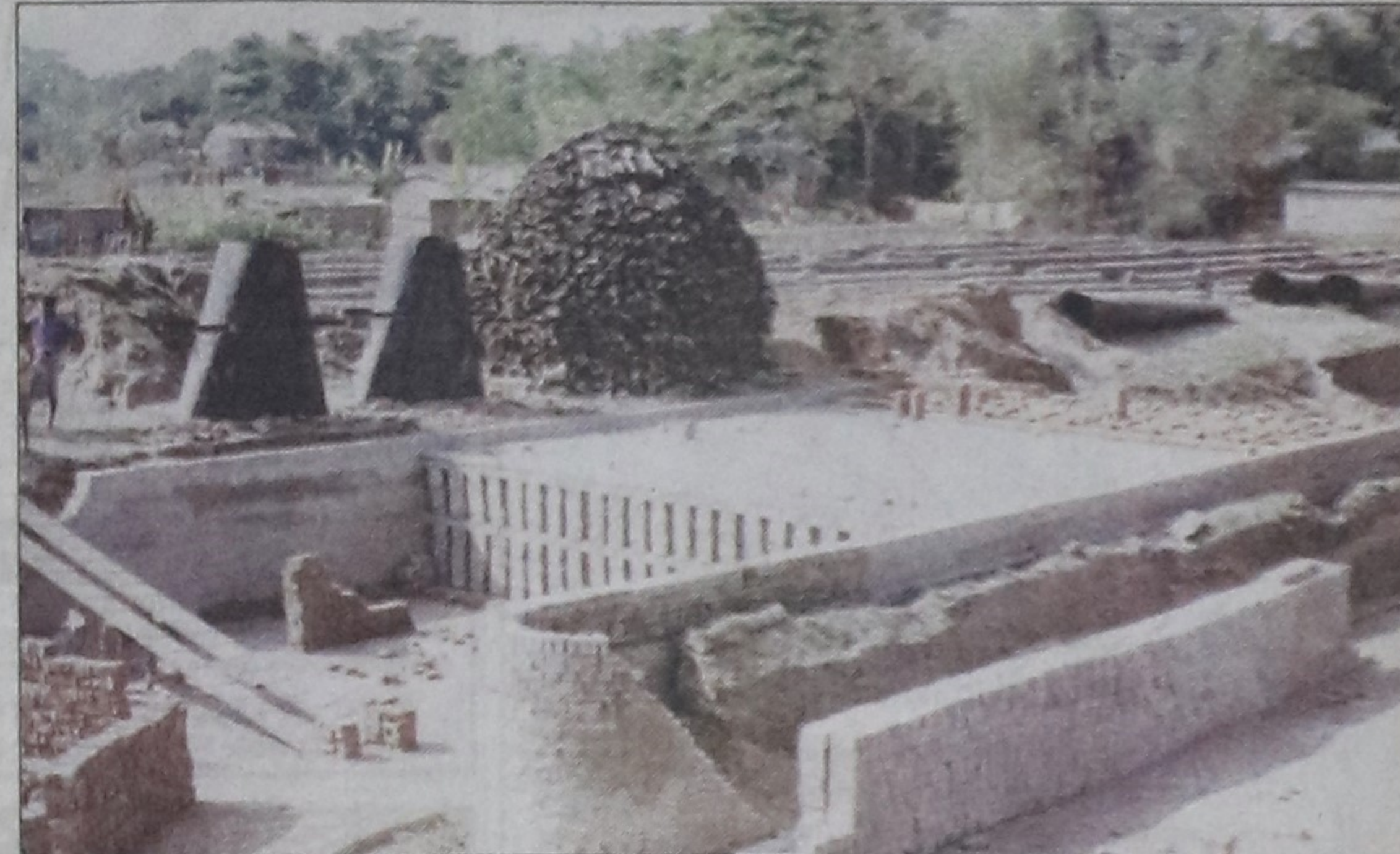
Ready to blaze... stacked coal and logs speak of Messrs Saudia Bricks' readiness to light its kiln anytime. The brick kiln on 3.5 acres of land surrounded by three villages in Nawabganj thana, 35 kilometres off the capital, has been given environmental clearance in defiance of all norms and regulations to start operations. Once it starts burning, human habitat and vegetation would come under serious threat. --Star photo by Amran Hossain
