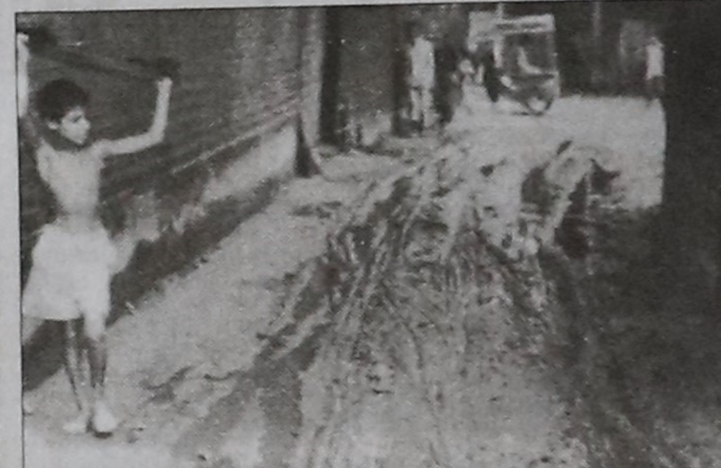
A muddy road caused by faulty drainage system in Ward Number 1 of Gaibandha Municipality. But there is no initiative from the authorities concerned for improving the situation. — Star photo
