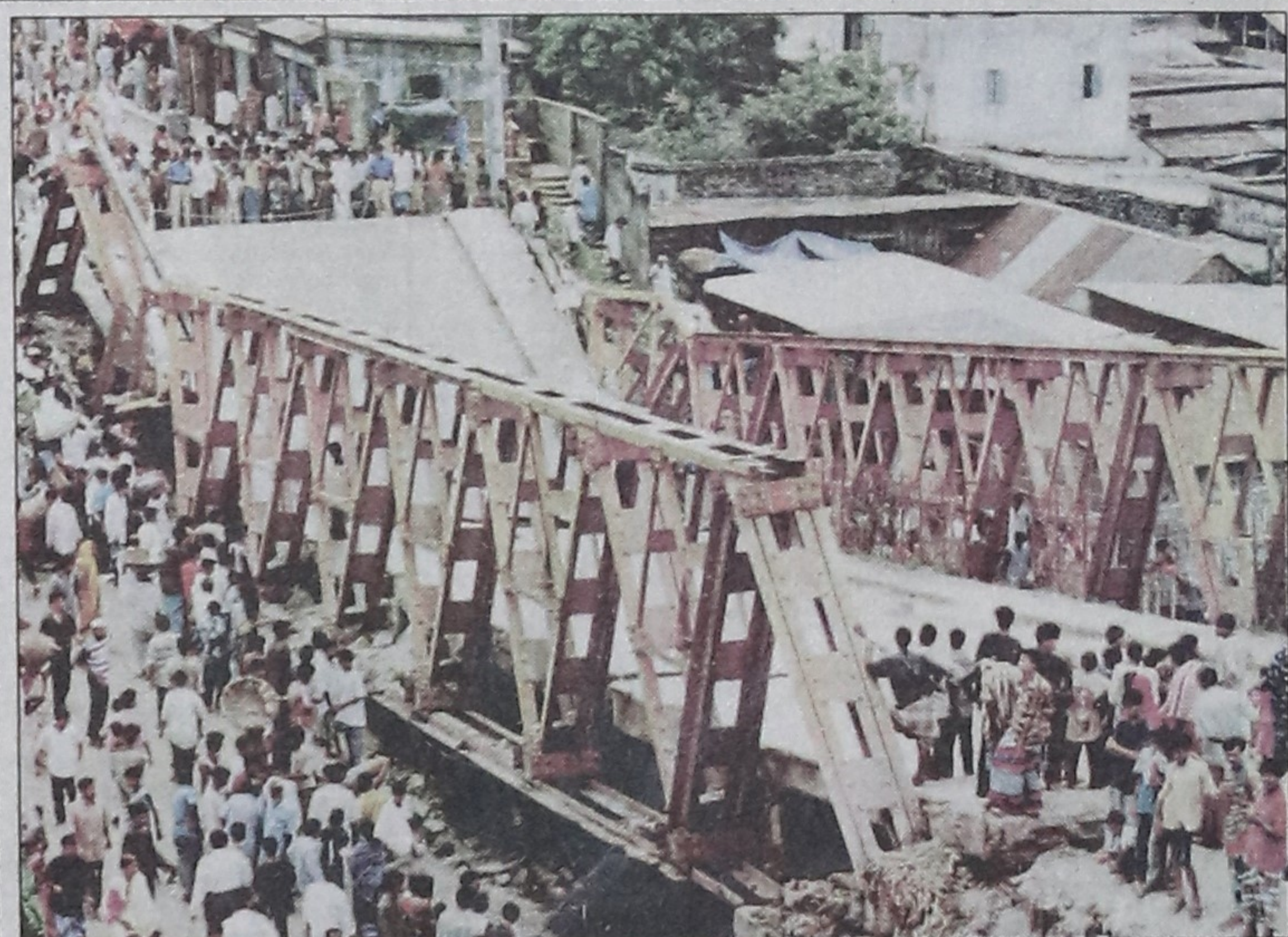
The run-down bridge over the city's Sutrapur canal, which has dried out for quite a long time, caved in yesterday morning while it was being dismantled. A new road is going to be built over the canal, making the steel structure redundant, anyway. — Star photo
