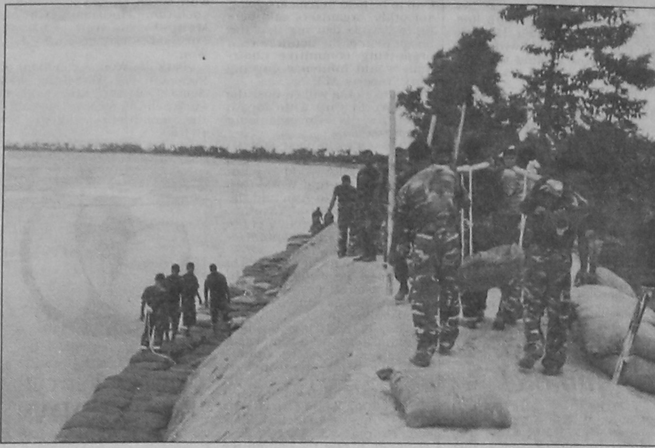
Members of Bangladesh Army repairing the erosion threatened Teesta embankment at Gangachhara in Rangpur.
