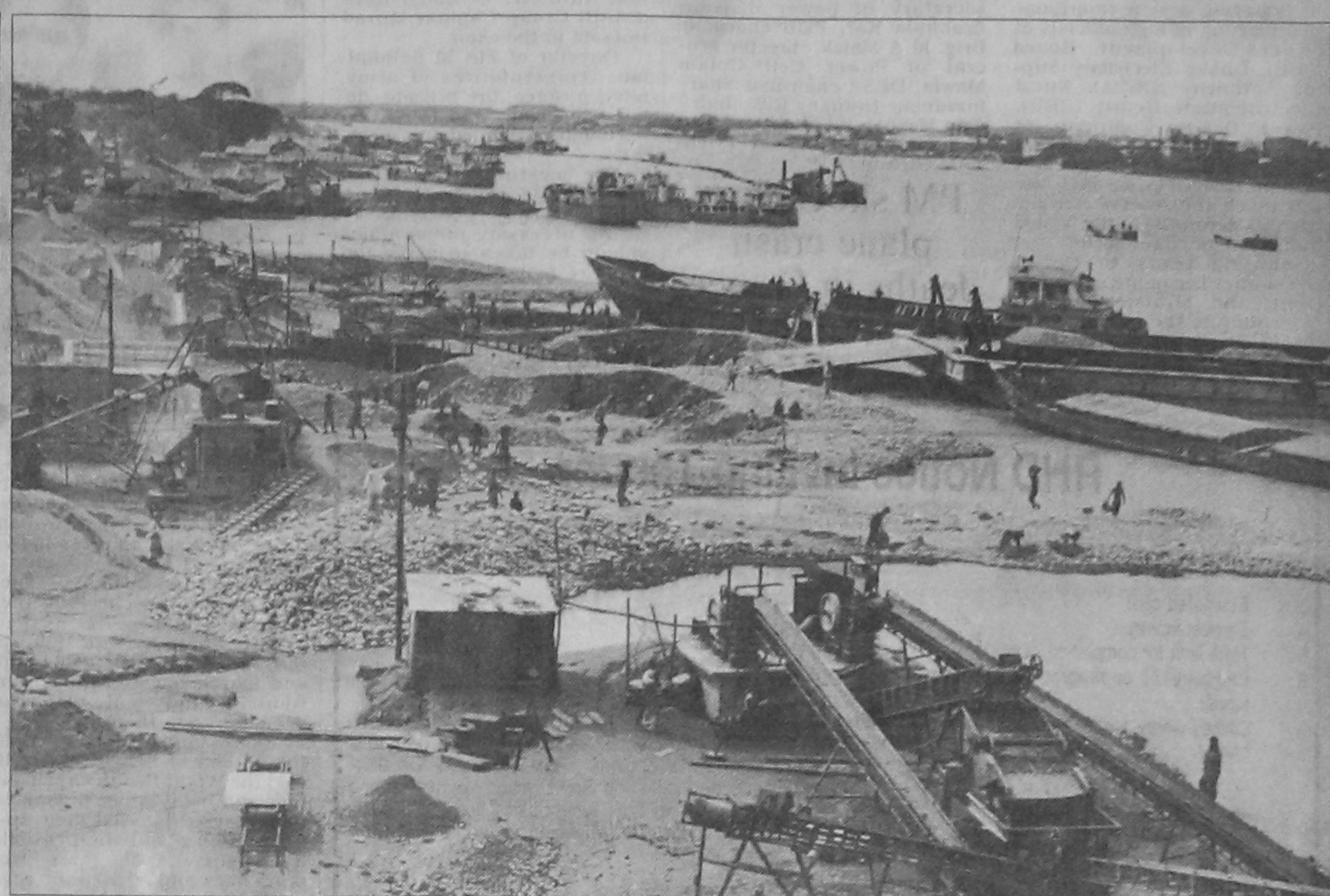
Encroachers do brisk business by gobbling up a big chunk of Shitalakkhya river close to Katchpur bridge. — Star photo
