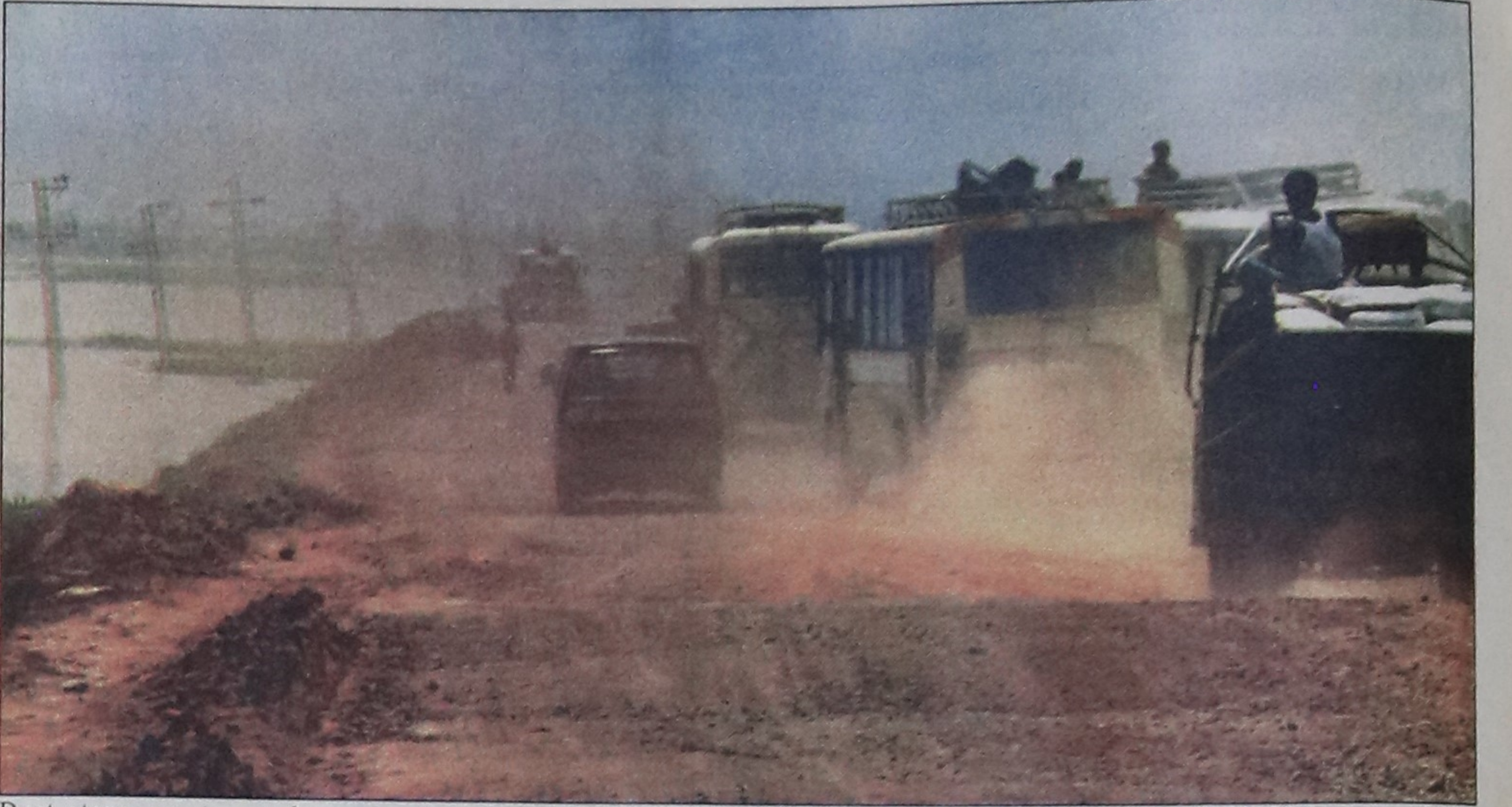
Dust storm greets people coming in or going out of the capital on Gabtali Aminbazar stretch of the highway under renovation for long. — Star photo by Anisur Rahman
