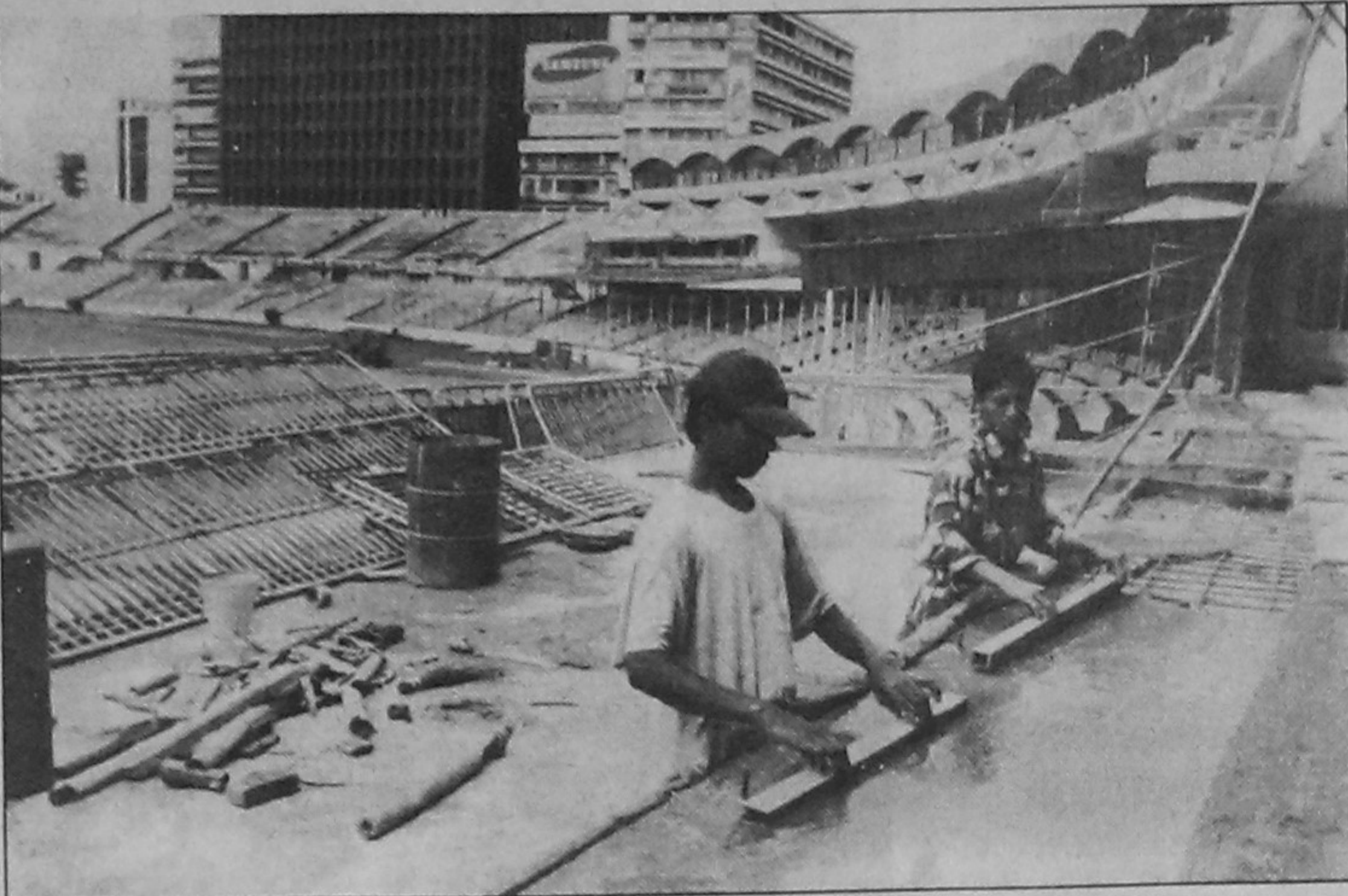
GETTING READY: Some renovation work is taking place at the Bangabandhu National Stadium ahead of the May 28-June 7 Pepsi Asia Cup. —Star photo
