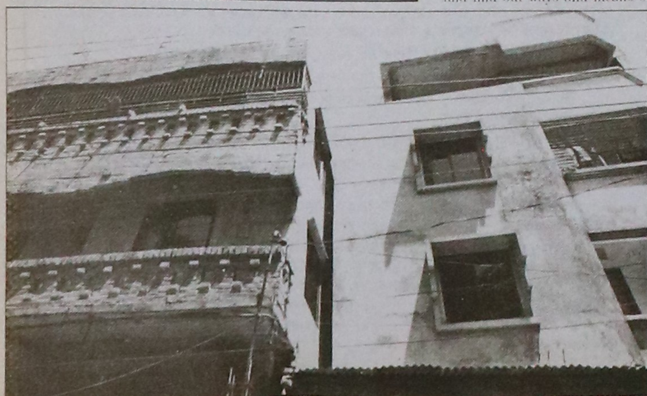
Leaving no space between buildings, blocking public thoroughfares with construction materials: Violation of rules, but who cares?
