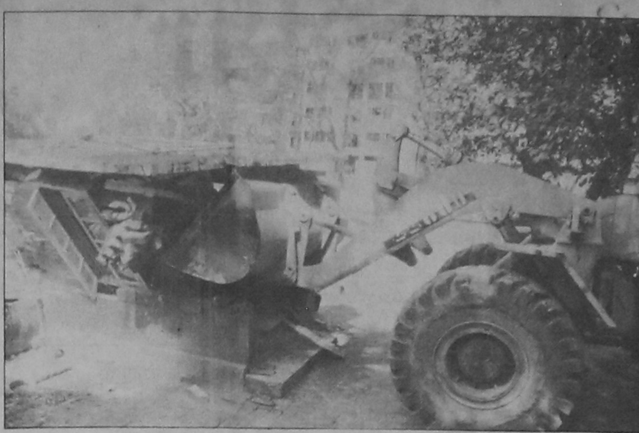
Dhaka City Corporation (DCC) and the Public Works Department (PWD) in a joint drive bulldozed illegal structures at Dhanmondi Lake area yesterday. — Star photo
