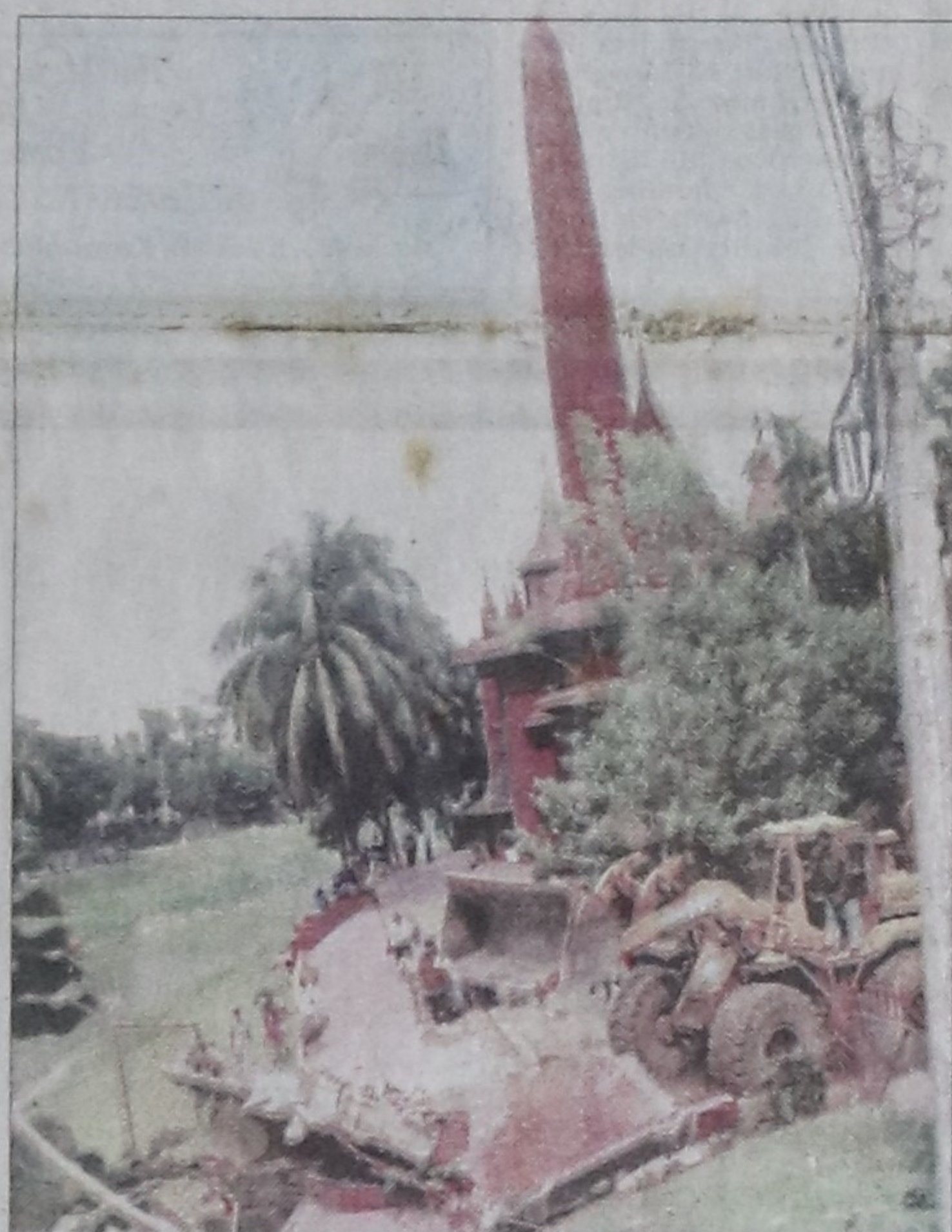
Bulldozers demolishing boundary walls of the palatial building of 'Sher-e-Khawja' at Dhanmondi yesterday. — Star photo
