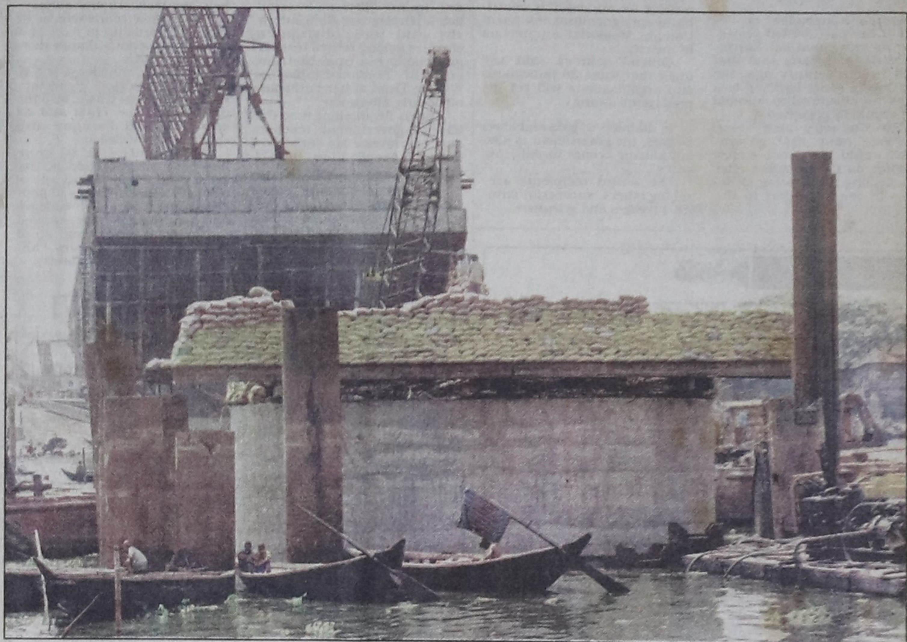
The second Buriganga Bridge was supposed to link Dhaka with Jinzira at Babu Bazar to ease traffic pressure. But that won't happen anytime soon. Work has been progressing at a snails pace, raising questions about the bridge's fate. — Star photo by AKM Mohsin
