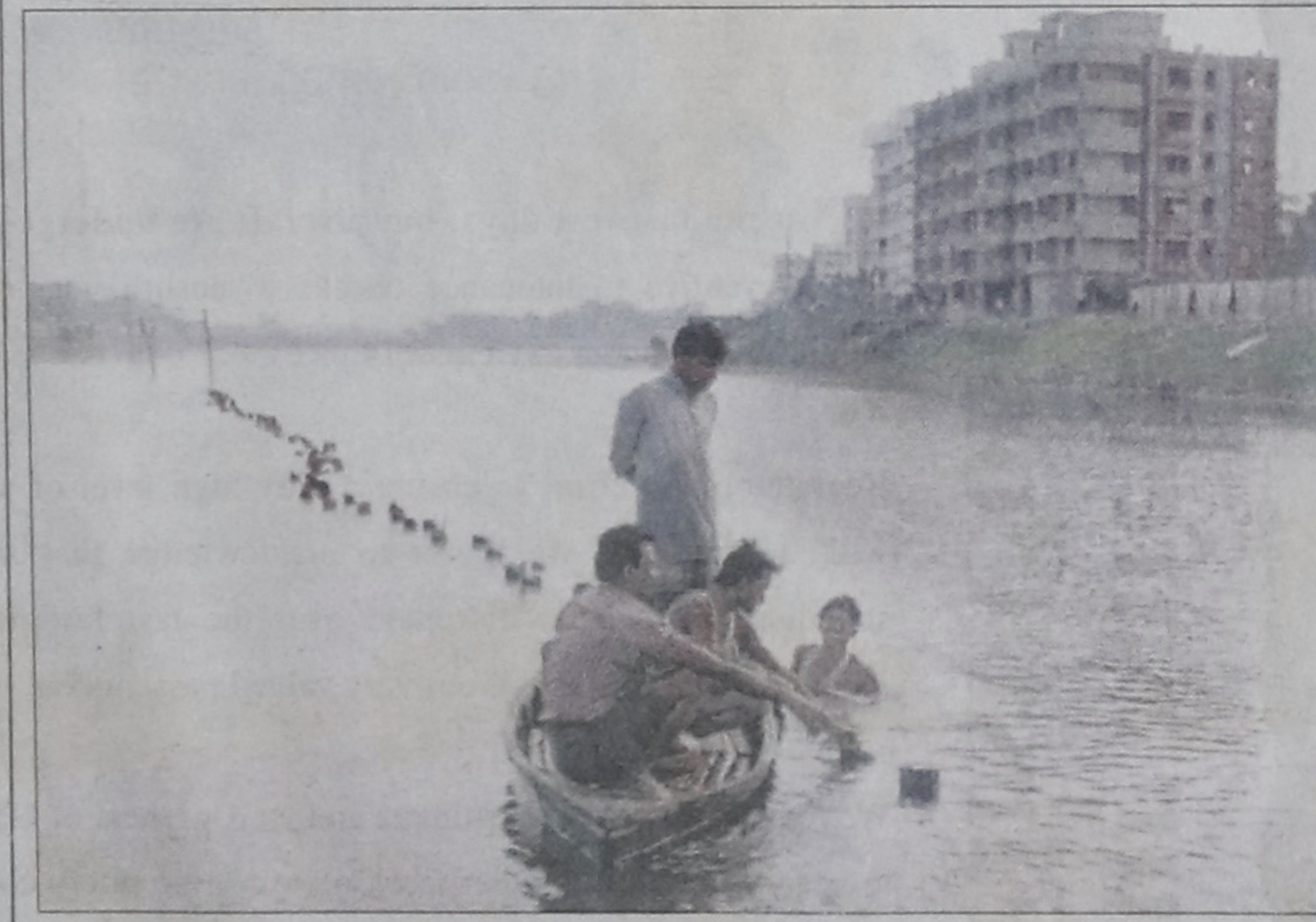
Wooden pillars sunk illegally in the Gulshan Lake by a real estate developer are being removed by Rajuk. This picture was taken yesterday. — Star photo
