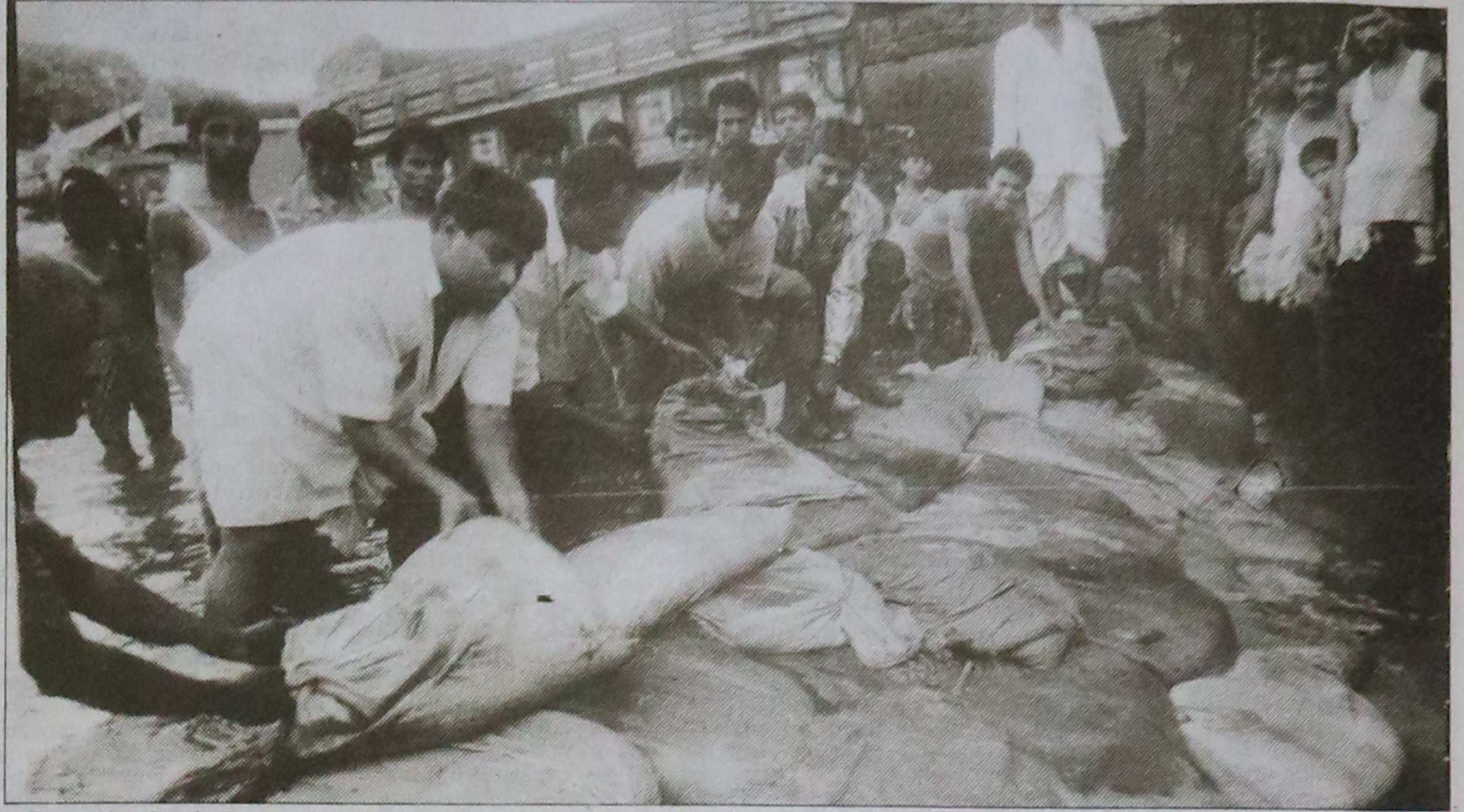
Affected by flood: Trying their best to save the eroding embankment
