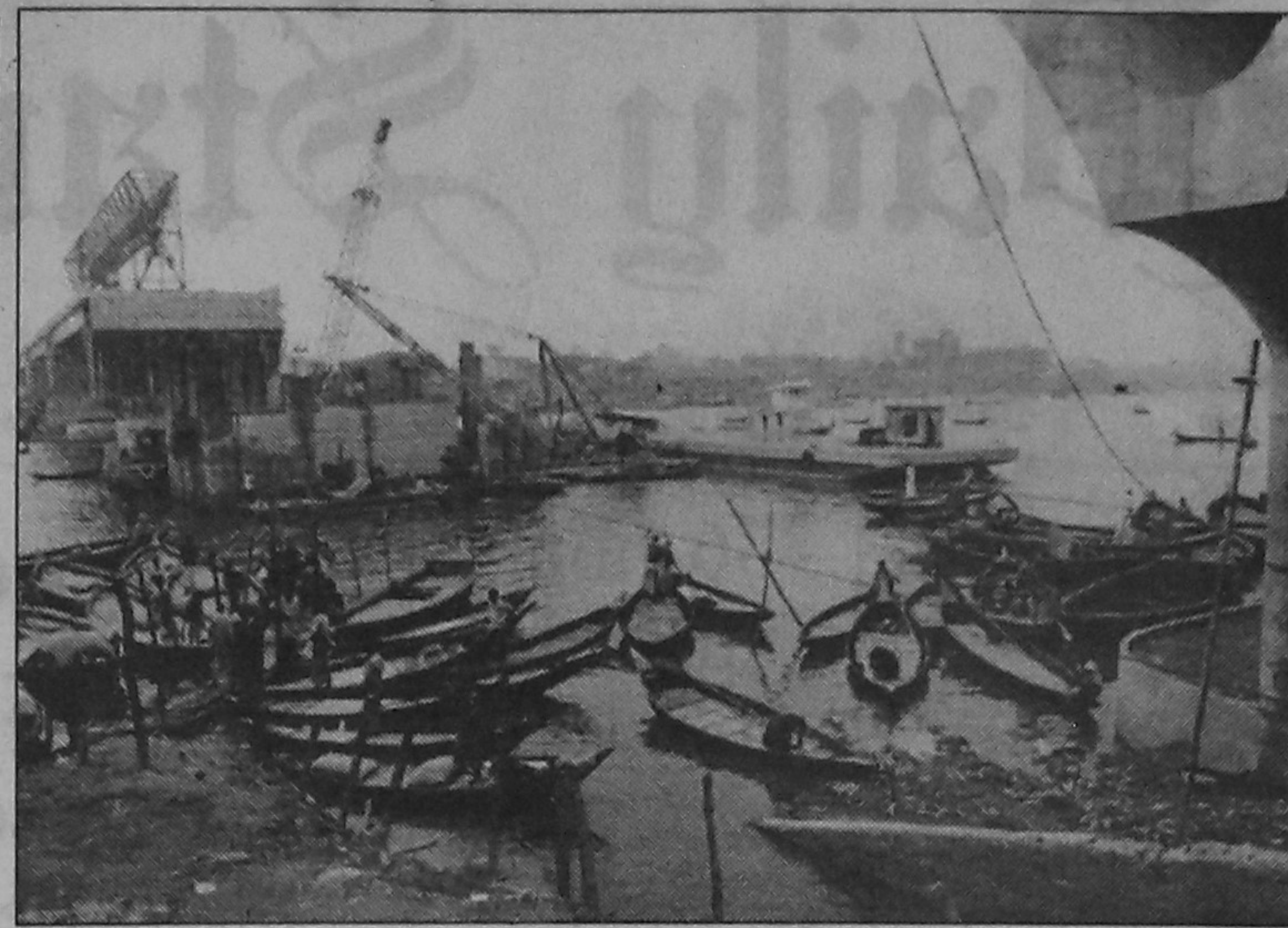
Construction of the 2nd bridge on River Buriganga is incomplete and no one yet knows when it's likely to be completed for use. — Star photo
